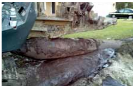
Pipe Boring Rig & 16" installation or highly treated sewer water polluting our rivers.
